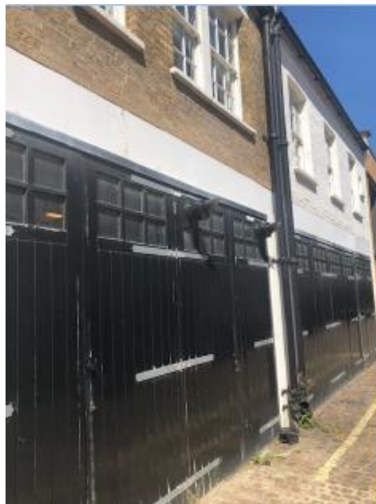
Detailed view of the flues as Installed
